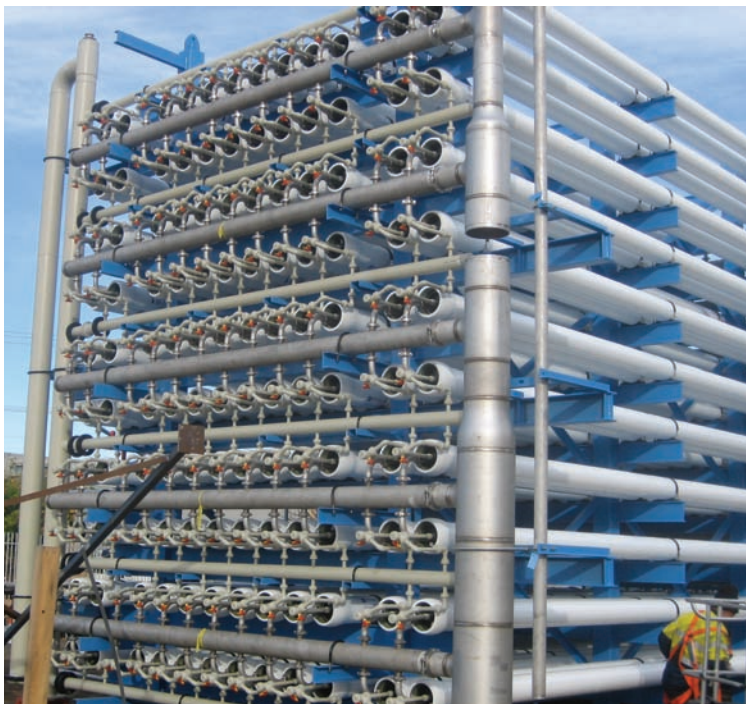
Reverse osmosis racks
