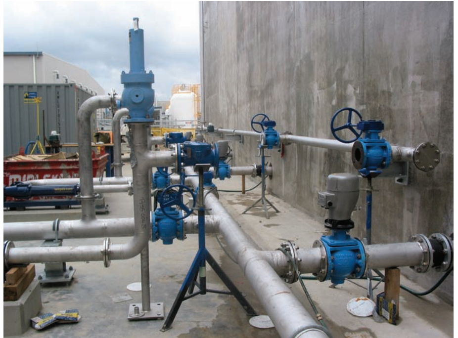
External pipes at the Bundamba Advanced Water Treatment Plant
